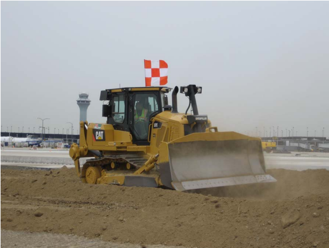
Photo 2 caption: The new diesel-electric hybrid Cat® D7E bulldozer moves earth at a work site on O'Hare International Airport's south airfield. The fuel-efficient bulldozer is one of many examples of how green technology is being implemented on the O'Hare Modernization Program. Photo credit: Chicago Department of Aviation
